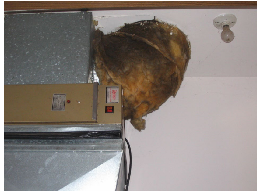
Signs of leakage
