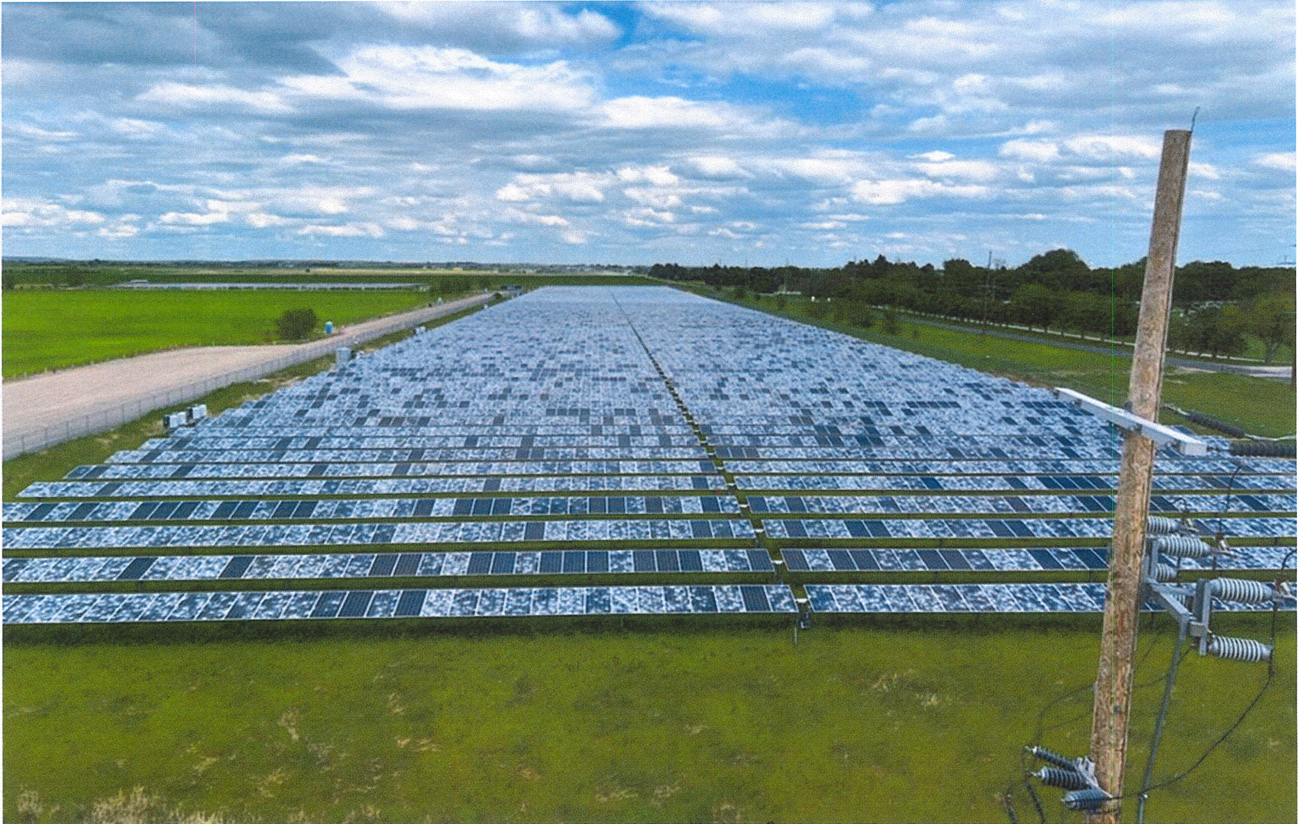
Hail severely damaged a solar farm in Scottsbluff, Nebraska on June 23, 2023. (Courtesy: Nebraska Public Power District)
