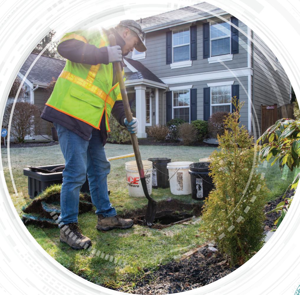
Installation of an advanced water meter for the Connect Up program.
