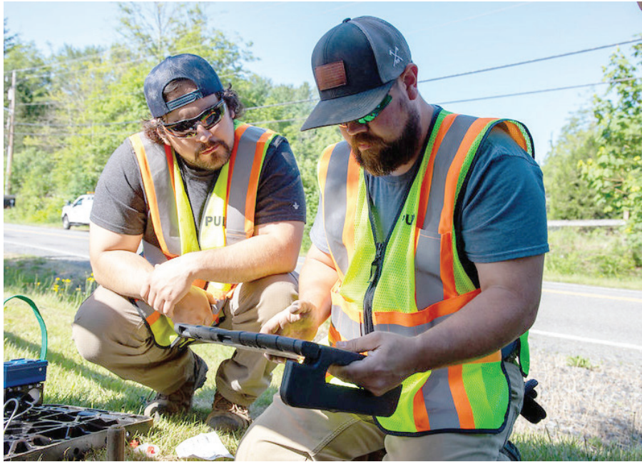
PUD staff install an advanced water meter for the Connect Up program.
