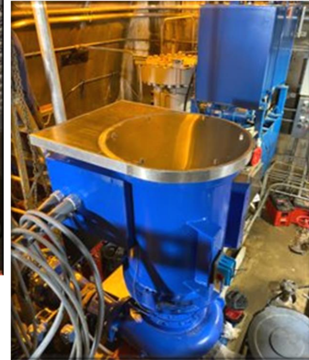
The new generator installed and operational
