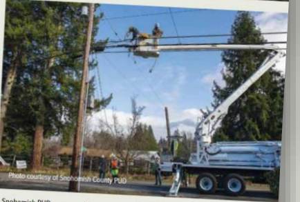
Snohomish PUD crews work to set a new utility pole (top) in the aftermath of a storm in January 2020. Snohomish County PUD crews work on restoring power after a significant windstorm in November 2022 (bottom).
