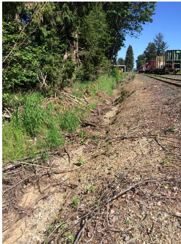
Photo 2. Ditch adjacent to site, May 10, 2016.
