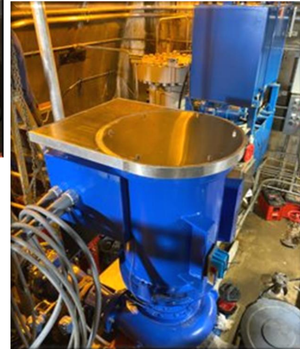
The new generator installed and operational
