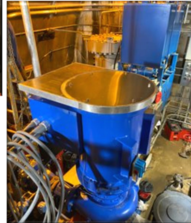
The new generator installed and commissioned
