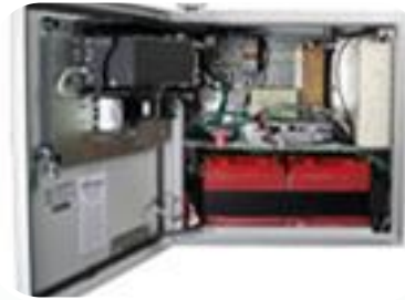
AMI Communications Network Deployment
