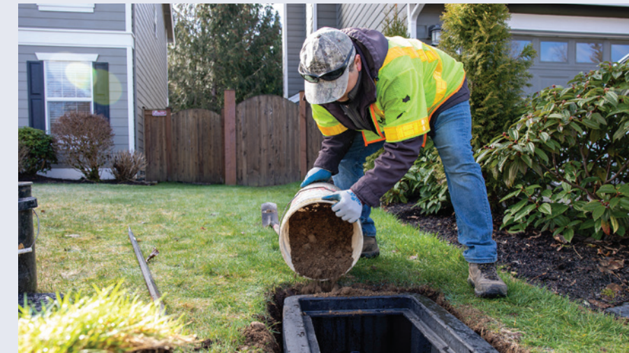
A water worker installing a new meter box in February. Groundwork is being laid for the utility's Connect Up advanced metering project.
