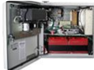
AMI Communications Network Deployment
