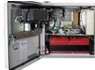
AMI Communications Network Deployment
