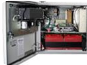
AMI Communications Network Deployment
