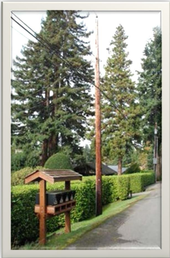
Typical Single-Phase Distribution
