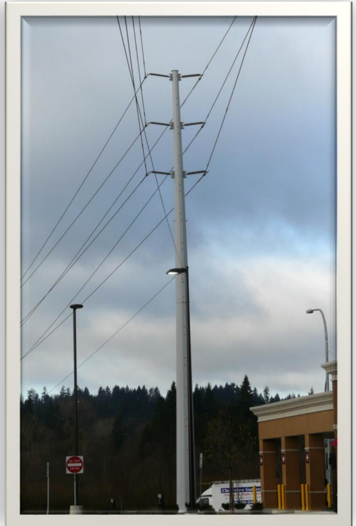
Typical 115kV Transmission Pole Steel
