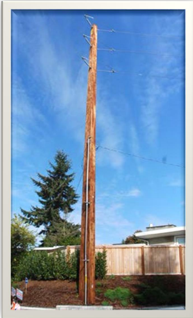
Typical 115kV Transmission Pole Glu-lam (laminated wood rectangular)
