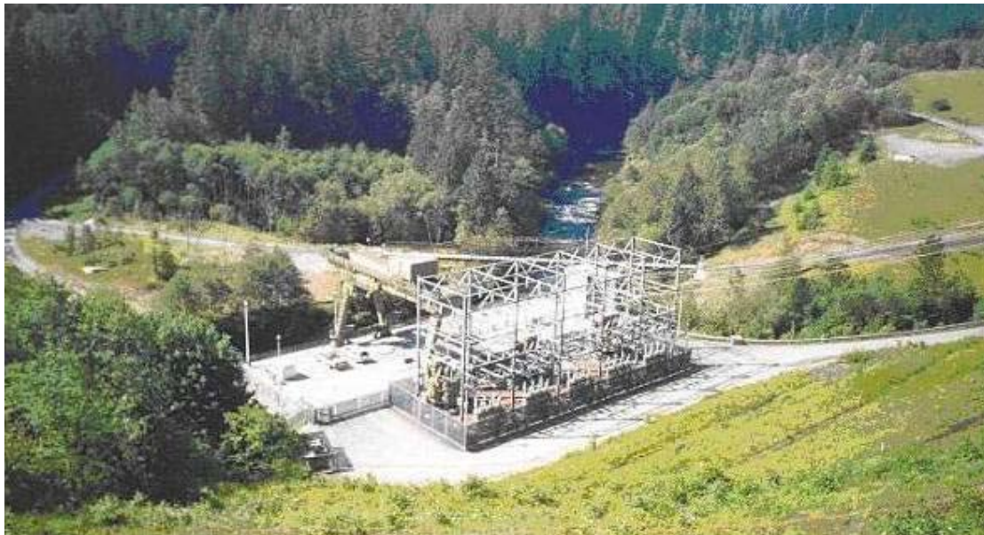
Figure 4 Jackson Hydroelectric Project powerhouse and switchyard.
